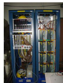
(b) New control rack.
