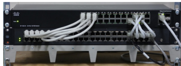
Figure 6: Ethernet switch and sync pulse injector.
