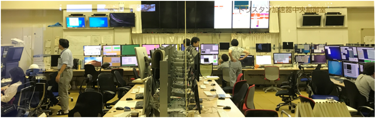
Figure 3: Picture of the main room at CCB. There are a lot of monitors for the operator consoles.
