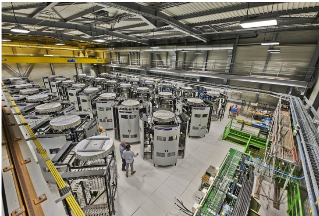
Figure 6: Amplifier hall with 32 towers.
