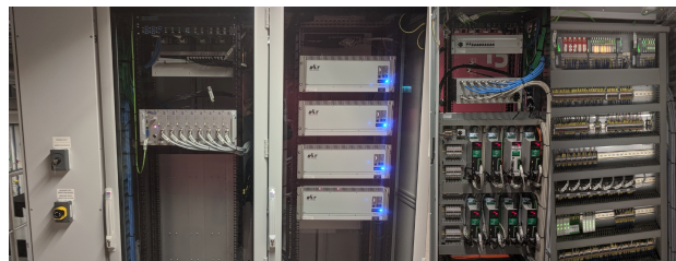
Figure 3: EPU control cabinets.
