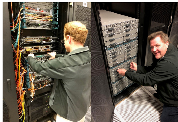
Figure 3: Before and after photos showing the difference homogenization makes to the infrastructure installation.
