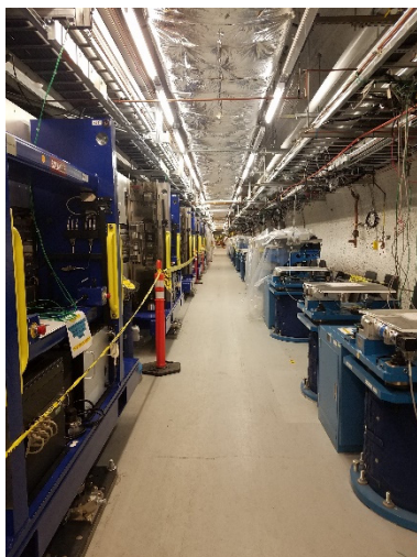
Figure 9: SLAC undulator hall. SXR undulators are visible on the left. HXR undulators and still empty girders are visible on the right. Beam direction will be into the page.
