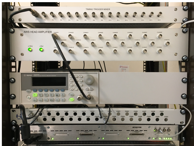
Figure 1: The demonstration system for the DWS connected to signals from various diagnostics systems at ISIS.
