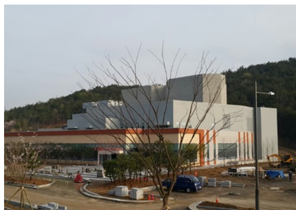
Figure 1: Site view of KHIMA treatment facility.
