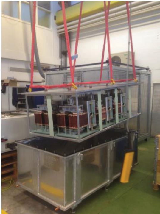
Figure 11: The Switched multi-level modulator prototype design and built at ESS. The prototypes is built for 120 kVA but the operational modulators will be for 660 kVA and will be provided as in-kind. Picture courtesy of Carlos Martins, ESS.
