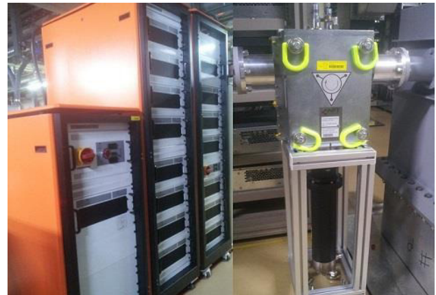
Figure 2: High power RF components (SSPA, Circulator, Dummy load).
