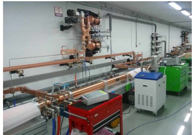
Figure 4: Photograph of the waveguide network system.
