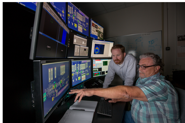
Figure 4: Operator work station, showing 9-screen control configuration, including the three main control screens and 6 system monitoring screens.
