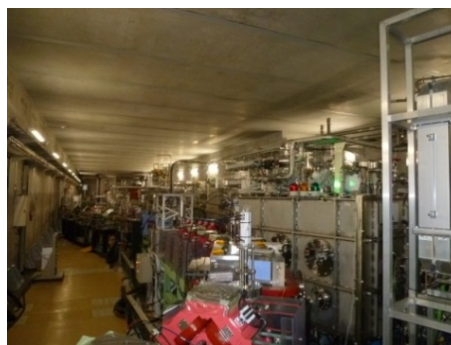
Figure 2: Injector cryomodule installed in beam line.
