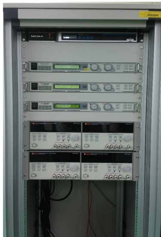
Figure 2: Magnet Power Supply and MOXA Terminal Server
