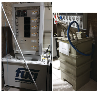
Figure 4: HV power supply and insulating transformer
