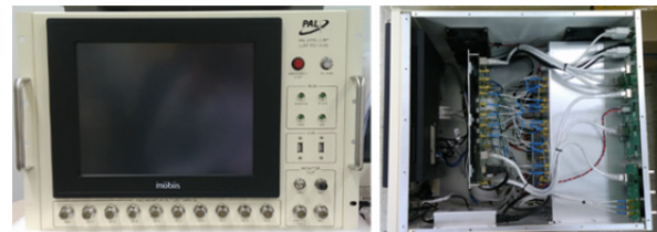
Figure 6: LLRF developed and installed for PAL-XFEL. Front view(left), and top view(right, cover is removed).
