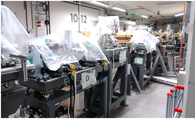
Figure 3: A Front End installed on the 1.5 GeV ring.
