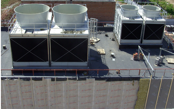
Figure 5: NSC KIPT Neutron Source secondary cooling loop building.
