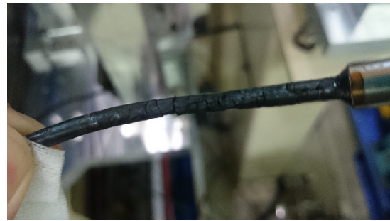
Figure 5: Temperature sensor cable damage by radiation.
