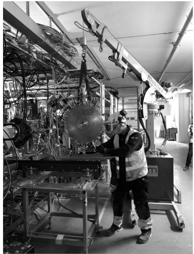
Figure 7: MEBT Assembly in the ESS LUND accelerator tunnel close up.
