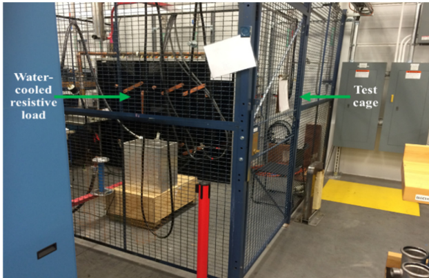
Figure 1: Test cage with water-cooled resistive load.
