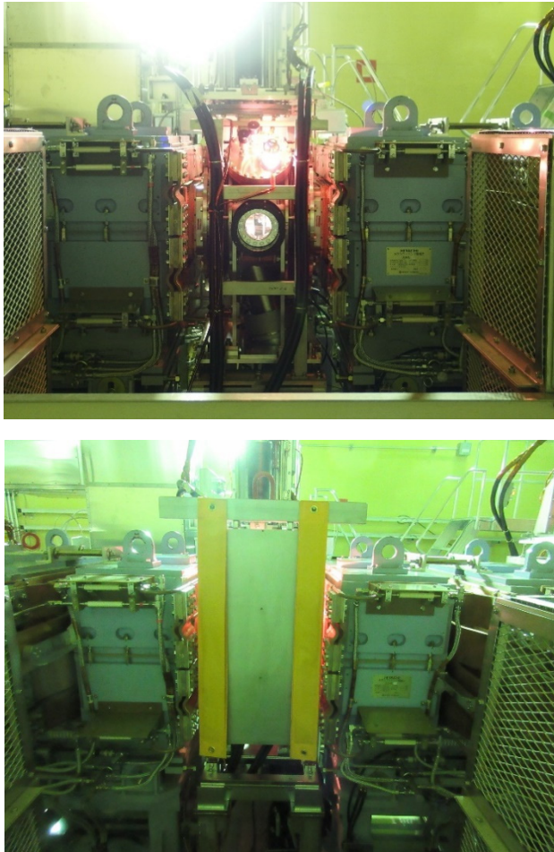
Figure 1: Injection point of RCS before (upper) and after (lower) the installation of temporary shielding.
