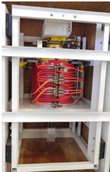
Figure 2: VKX8311A klystron during the unpackage.
