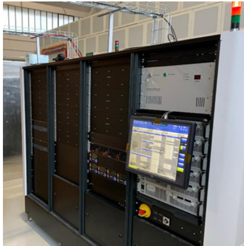
Figure 1: Solid state modulator installed near the TEX bunker.
