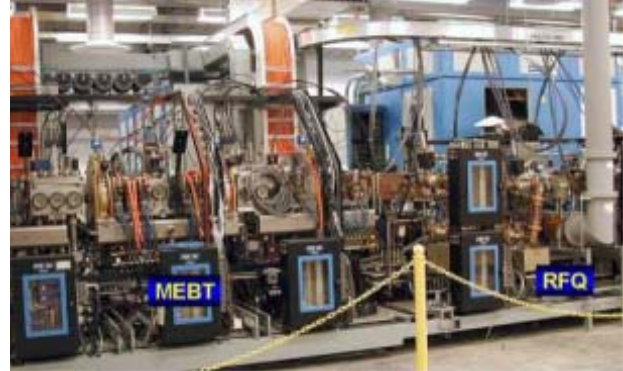
Figure 4: Front-End System installed at SNS-ORNL.
