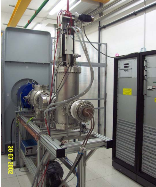
Figure 3: Trips source with EMU installed.
