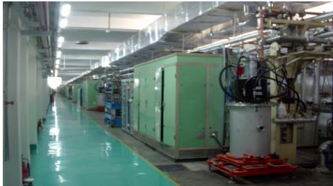
Figure 3: Picture of BEPCII klystron gallery.
