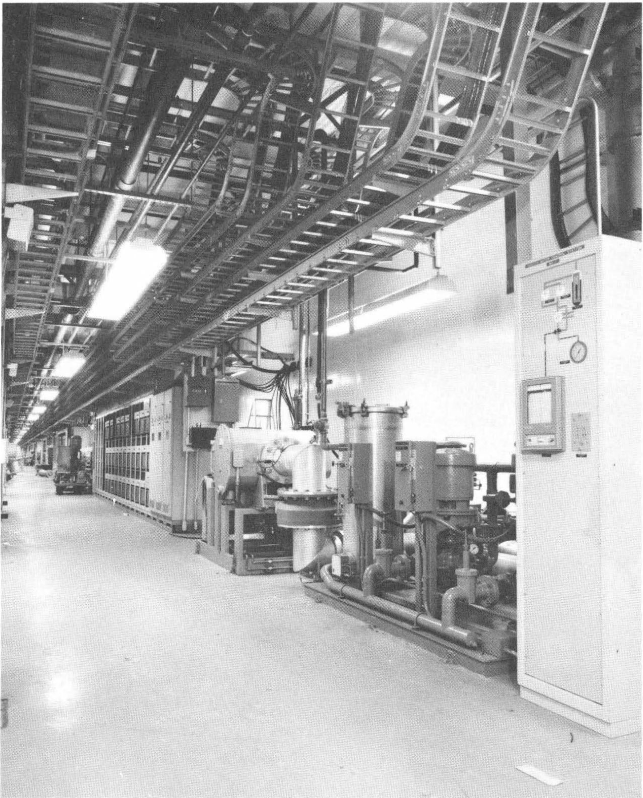
Fig. 10. The lower equipment bay.
