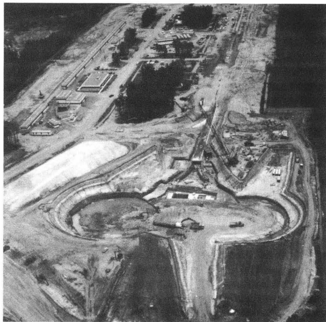
Figure 2. CEBAF civil construction progress, July 1990. End station excavation in foreground; accelerator surface buildings in background; injector service building near the center left edge.
