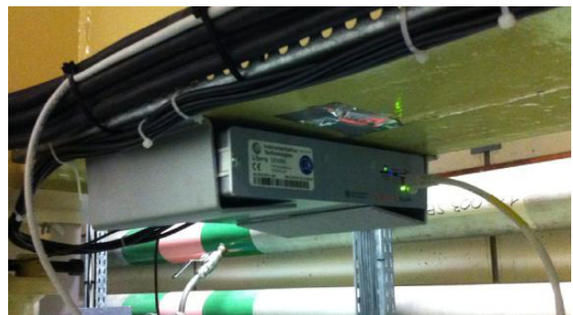
Figure 9: Spark ER installed at ESRF.
