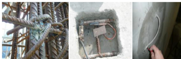
Figure 5: Welding of the iron frameworks and implementation of connection to link processes and cable trays to the global ground.
