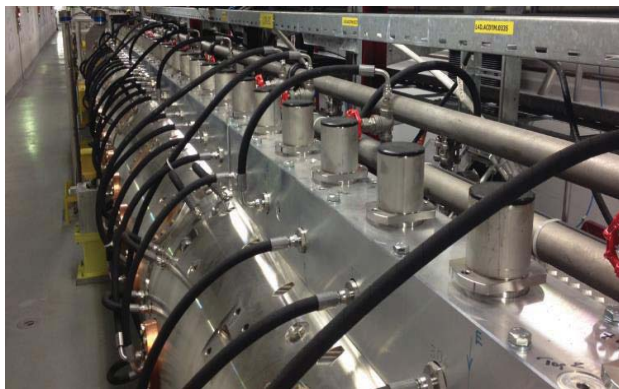
Figure 2: DTL tank3 drift tube alignment girder.
