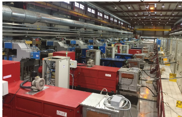
Figure 2: View of CERN Linac4 klystron gallery.
