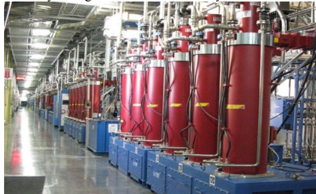
Figure 5: SNS klystron gallery, klystrons CPI VKP-8291B.
