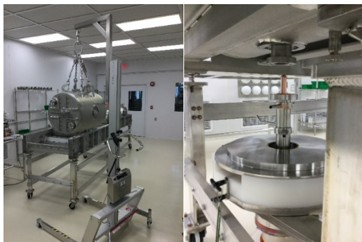
Figure 5: \beta=0.53 cavity ready to install on coldmass and FPC installation to coldmass.
