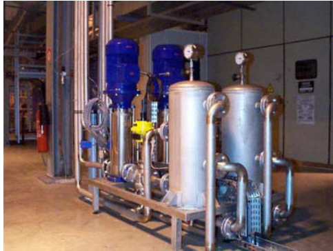
Figure 1: Two of the ESRF cavity cooling racks.
