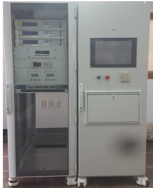
Figure 4: PLC rack of QWR cryomodule.
