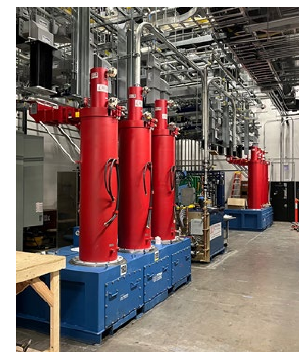
New 700 kW klystrons installed
