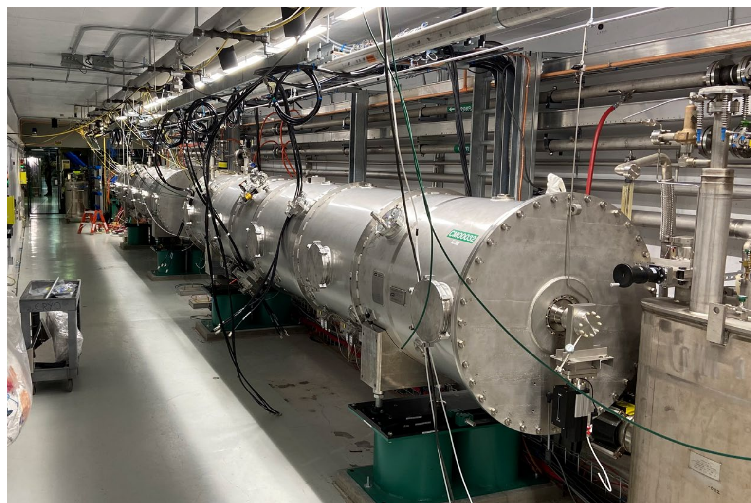
The first two cryomodules mounted on their stands in the Linac enclosure
