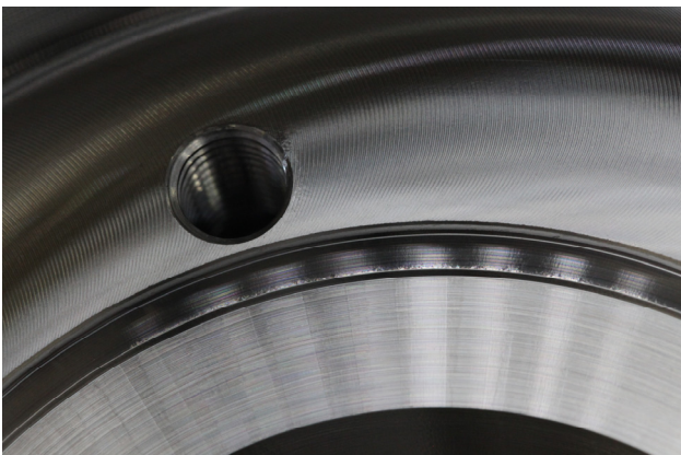
Figure 18: Last picture documents the orange skin micro damages on the scintillation screen monitor vacuum chambers for E-XFEL project.
