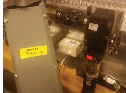
Figure 14: Mounted tilt meter.
