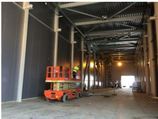
Figure 12: Cold box hall.
