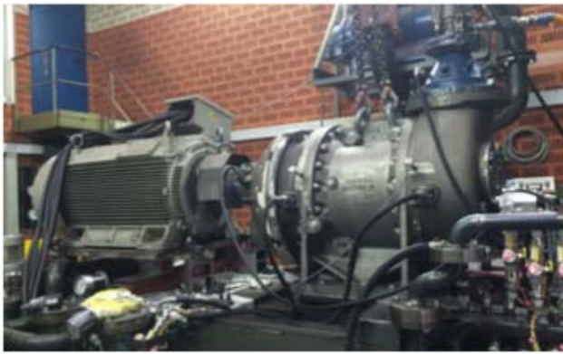
Figure 8: Factory acceptance testing of one of the ACCP helium compressors at Aerzen.
