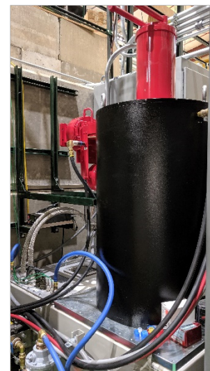
Figure 2: Picture of klystron, focusing solenoid & High voltage transformer tank assembly.
