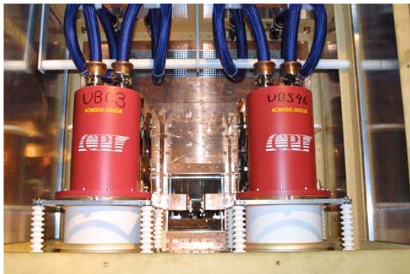
Figure 4: Inside of 1.2MW final stage amplifier
