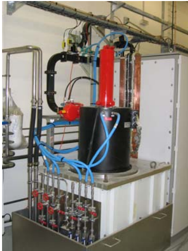
Figure 6: A klystron with the oil tank and the focusing in the RF hall before installing the lead protection.
