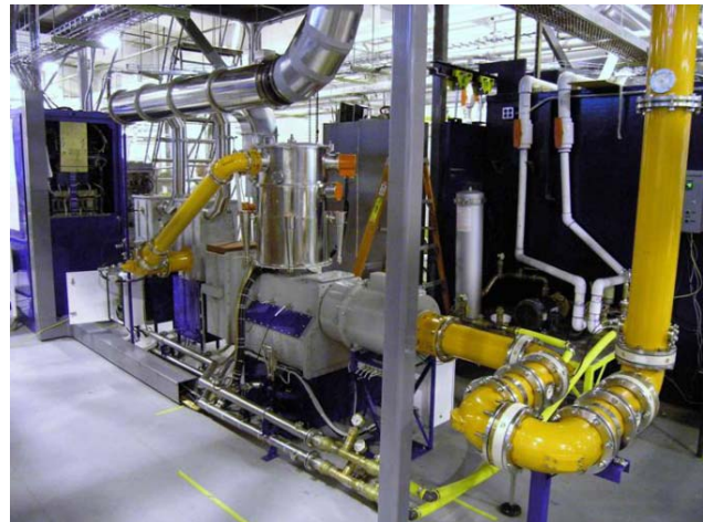
Figure 1: New DFELL generator.
