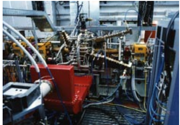
Figure 2: The RF cavity installed in the positron ring.
