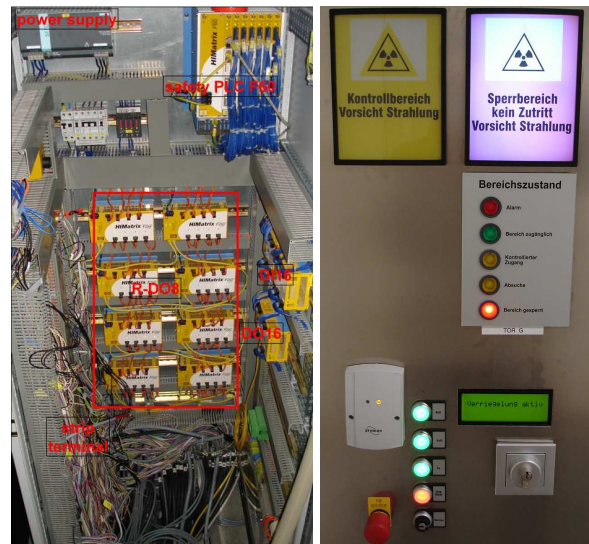
Figure 2: Layout of the central PSS rack (left) and the display at the shielding doors (right).
