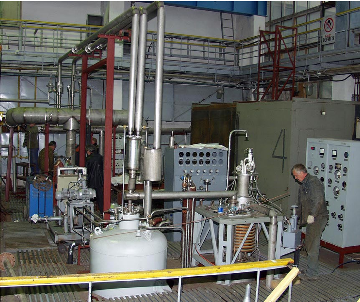
Fig. 3: Helium refrigerator, large vacuum heat exchanger and liquid helium bath (last two in the background) during erection.
