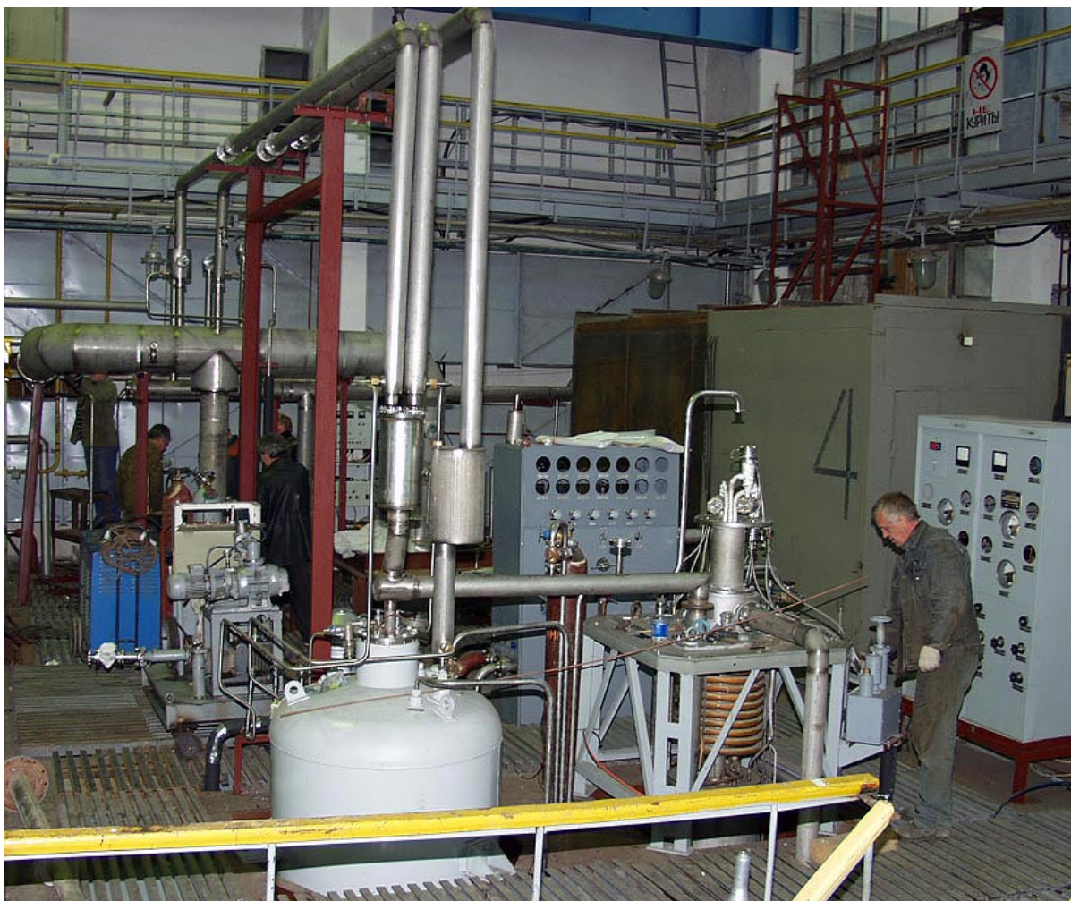
Figure 3: Helium refrigerator, large vacuum heat exchanger and liquid helium bath (last two in the background) during erection
