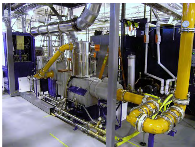
Fig. 1: New DFELL generator
