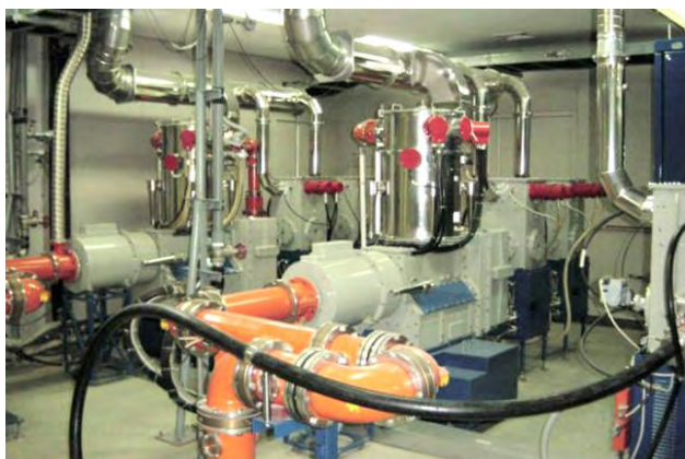
Fig. 3: RF generators 176 MHz
