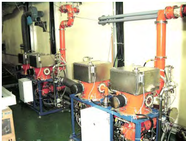
Fig. 6: RF generators 352 MHz
